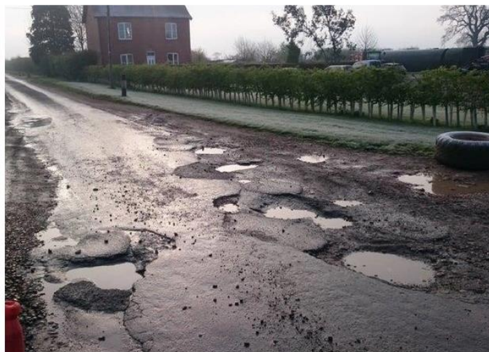
Fig.1 Road with Potholes
